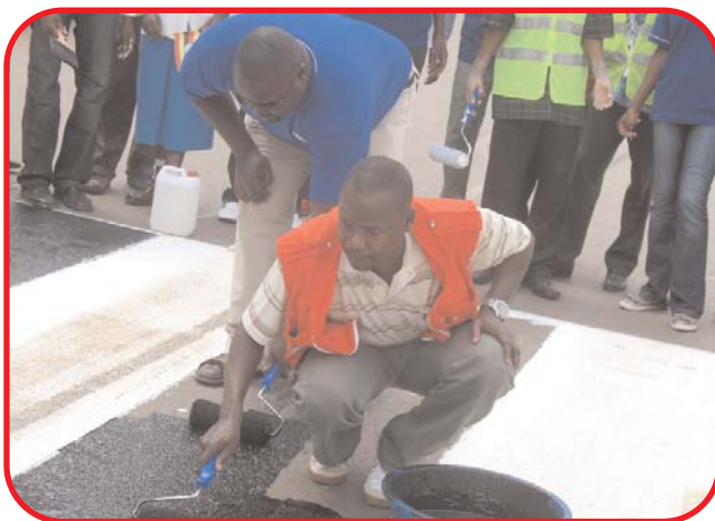
URCS Acting Secretary Michael Nataka and NSSF Managing Director Chandi Jamwa paint the zebra crossing at Post Office on Kampala Road.
